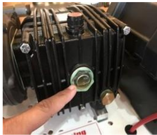
Figure # 2 – Oil Level in Pressure Pump
