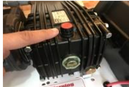
Figure # 6 – Pump Oil Fill Port
